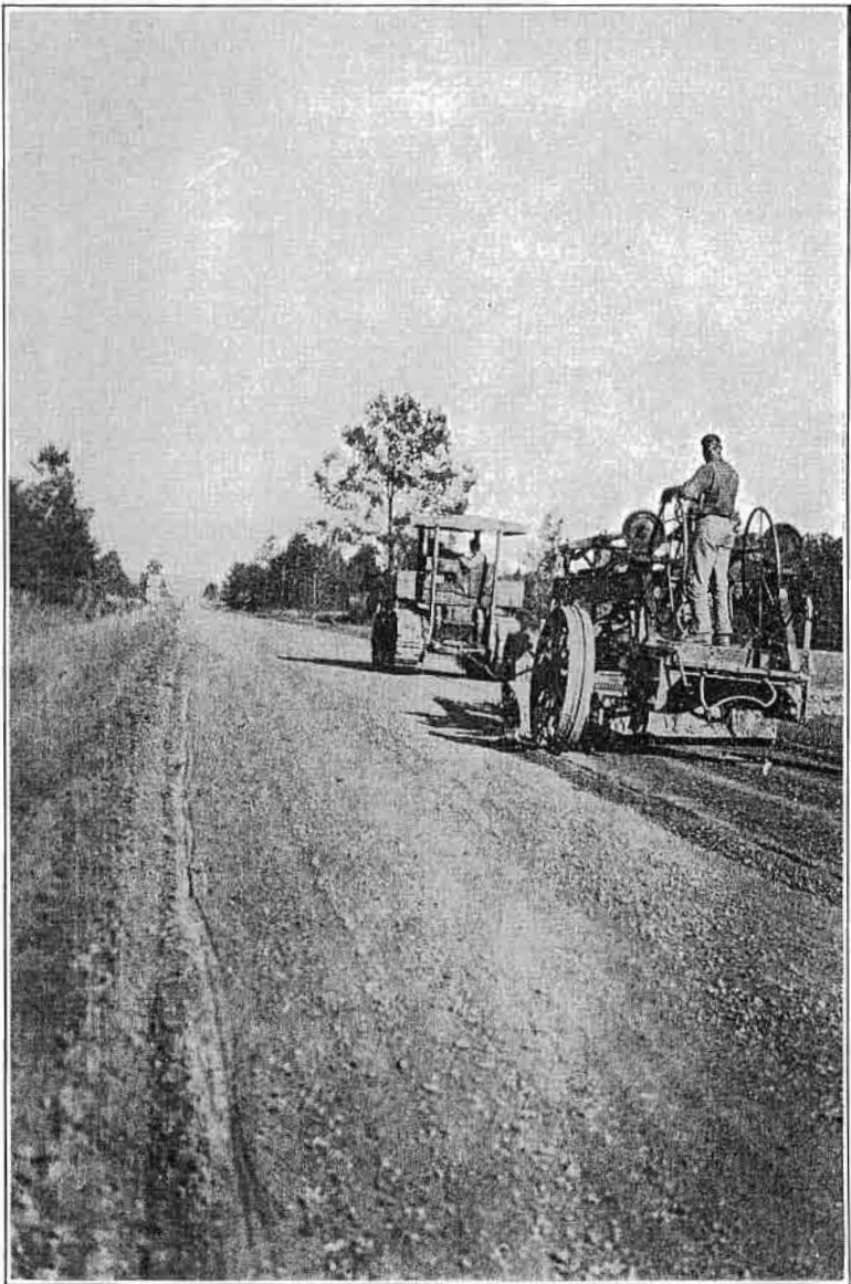
Another View of State Highway Department Equipment at Work on the Maintenance of Gravel Roads. This view was taken on the Van Buren-Alma Road in Crawford County.
