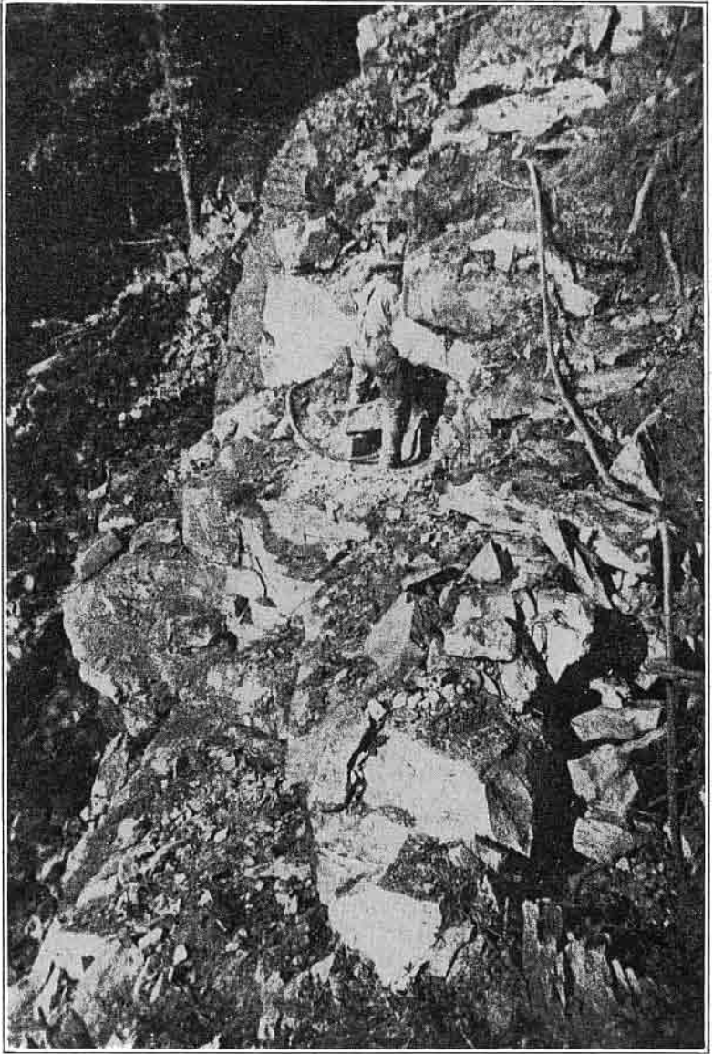
A difficult, rocky ledge on the center line of the New Highway under construction between Western Grove and Lurton in Newton County.
