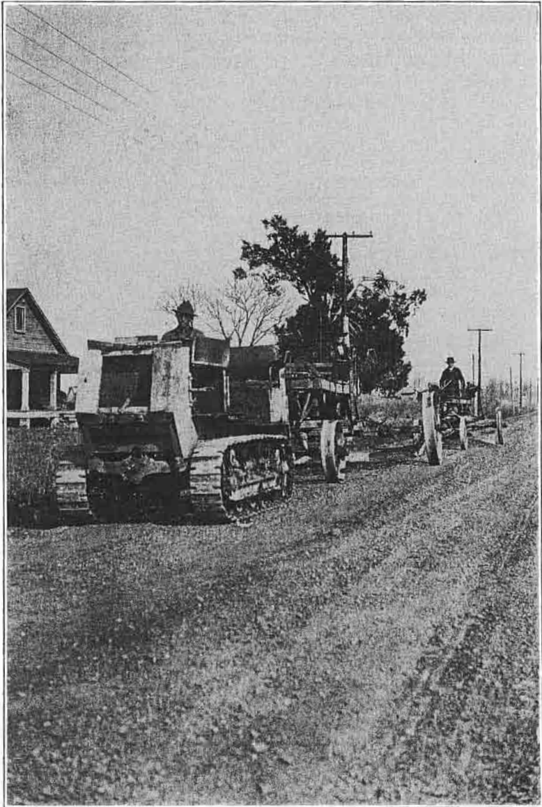
A Five-Ton Caterpillar Tractor, Two-Grader Maintenance Outfit at work on gravel roads on the Highway System in Crittenden County. This has been a very serviceable unit for maintenance work.
